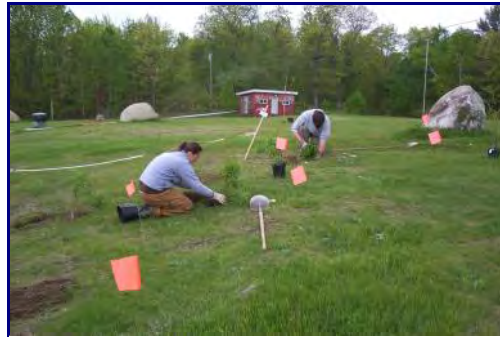
The Cooperative Extension's Buffer Brigade provided the labor for installing the buffer demonstration at Lakeside Landing.
